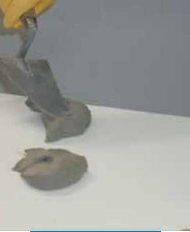
Applying Mapetherm AR1 on the back of the panel and spot bonding with a trowel
