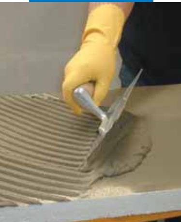
Applying Mapetherm AR1 on the back of the panel with a notched trowel
