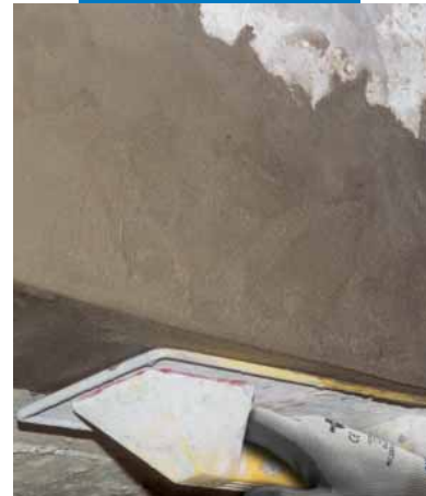
Patch-work of a concrete beam
