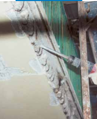
Restoring the front of the concrete slab of a balcony: preparing the substrate
